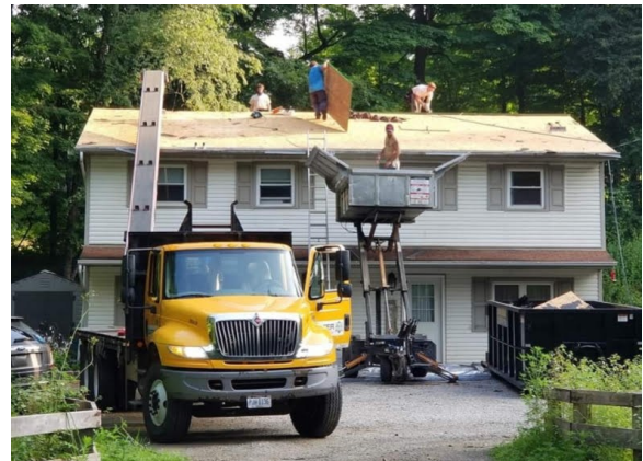
Badly-needed Roof Repair...$8,900
